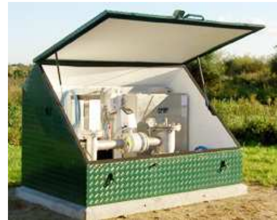
Bore well station
